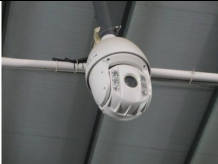
CCTV camera at material warehouse 原材料仓库闭路监控设备
