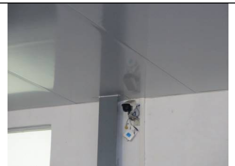
CCTV camera at assembly workshop 装配车间闭路监控设备
