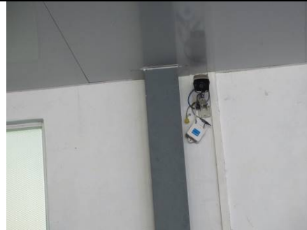
CCTV camera at packaging workshop 包装车间闭路监控设备
