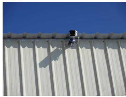
CCTV Camera at loading area 装卸货区闭路监控设备
