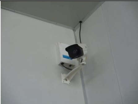
CCTV camera at Laminating workshop 复膜车间闭路监控设备
