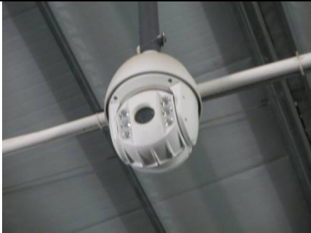
CCTV camera at printing workshop 印刷车间闭路监控设备
