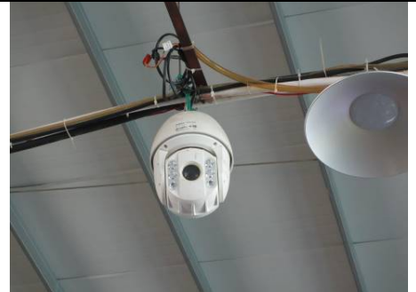
CCTV camera at bag making workshop 制袋车间闭路监控设备
