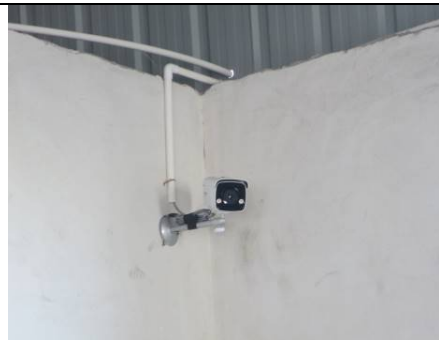
CCTV camera at finished goods warehouse 成品仓库闭路监控设备
