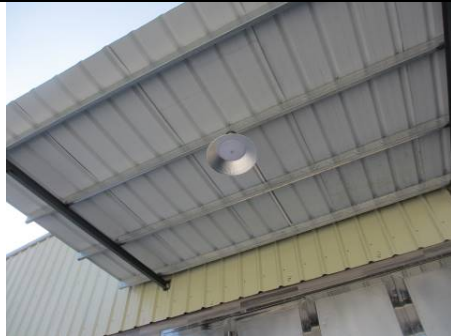
Floodlight at loading area 装卸货区照明灯
