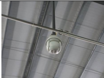
CCTV camera at cutting workshop 裁切车间闭路监控设备
