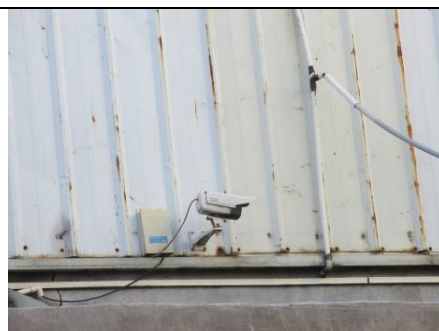
CCTV camera at factory Wall 工厂围墙闭路监控设备
