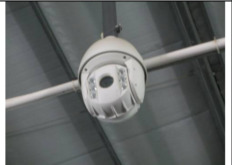
CCTV camera at slaking workshop 熟化车间闭路监控设备
