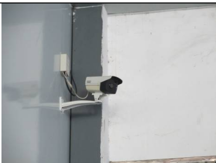
CCTV camera at Punch Machinery workshop 冲床车间闭路监控设备
