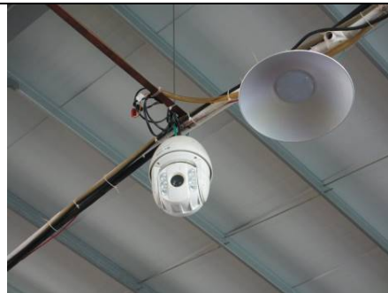
CCTV camera at balloon hanging workshop 挂球车间闭路监控设备
