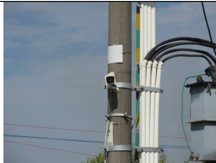
CCTV camera at factory gate 工厂大门闭路监控设备
